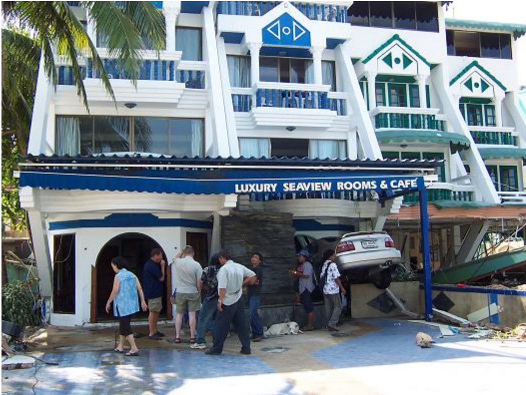
Cars, steel, and other debris slammed into buildings over a two hour period (photo Dec. 27)
